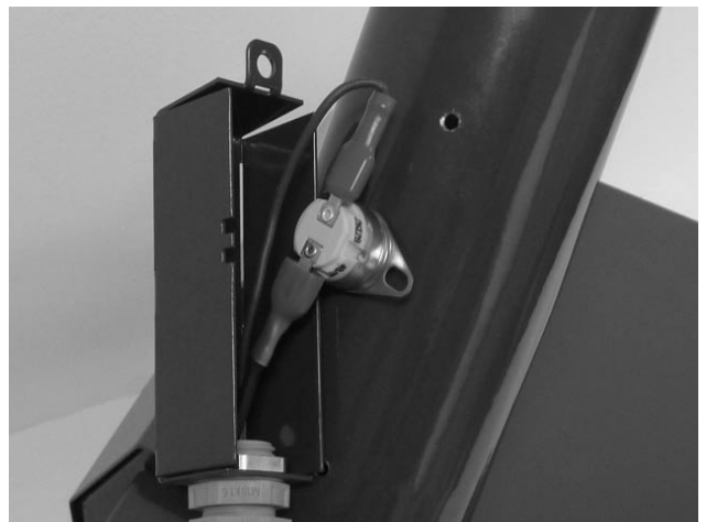
Fig. 10 - Safety thermostat on the pellet supply pipe, 95 °C
