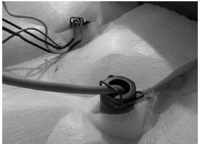
Fig. 16 – View of the water temperature sensor TK in the boiler pocket, DxxP type
